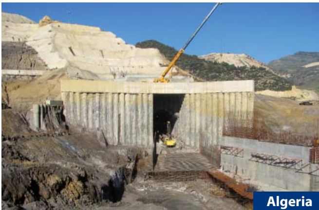
Project Djedra Dam Services Design; Supervision; preparation of the detailed design, technical assistance and supervision over construction; Client ANBT (Agence nationale des barages et transferts)
